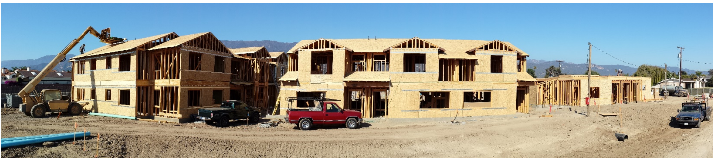
Photo: Courtesy of Peoples' Self-Help Housing. Construction of the 43-unit Casa de Las Flores project is underway in Carpinteria.
